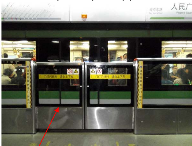
A barrier sliding door is closed until a train is at a full stop
