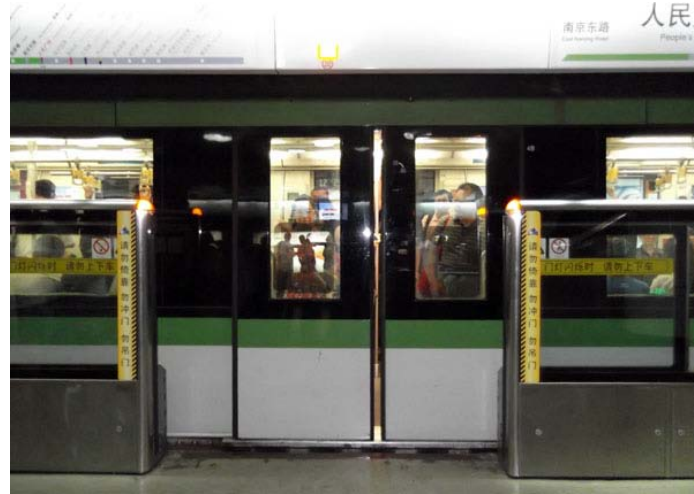
A barrier sliding door is open after a train is at a full stop
